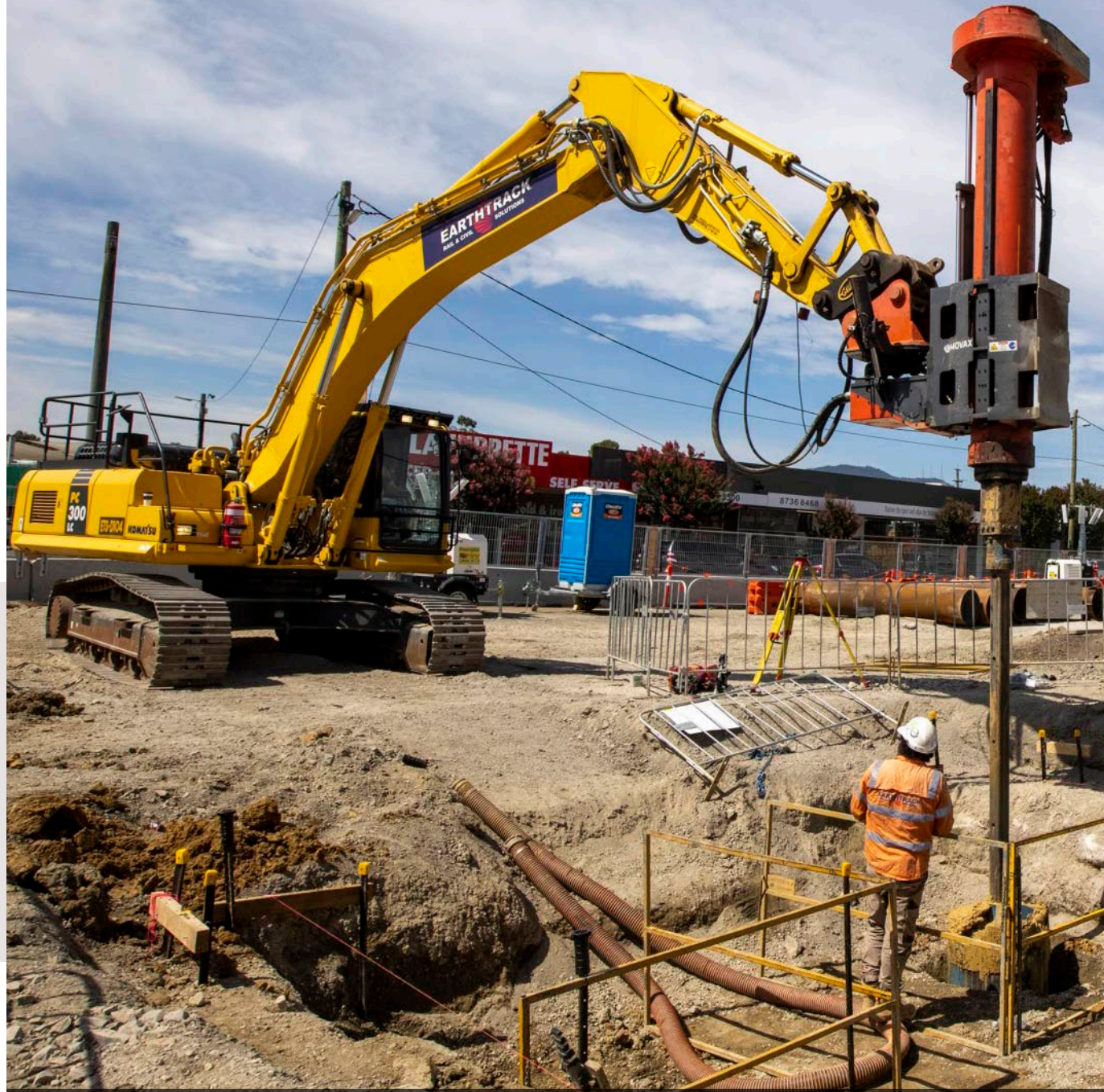
Image 9. Level crossing removal works in Lilydale. Credit: © State of Victoria (Level Crossing Removal Project)
